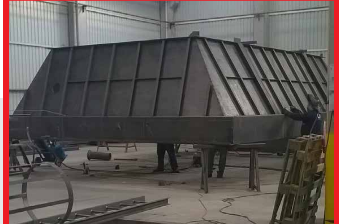
Cement Plant Filter Hopper
